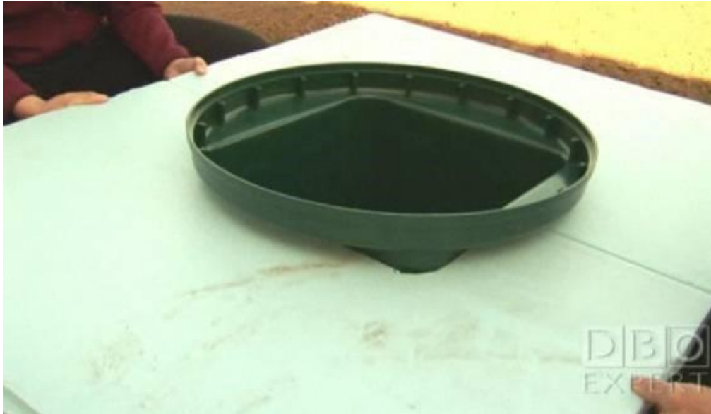
Figure 75. Insulation around a distribution box
